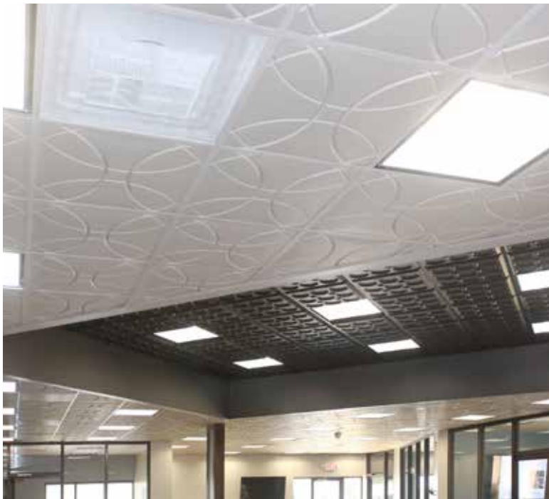
The interior features a large open-office area, surrounded by a few private offices and conference rooms. The room is visually centered by a graphic design of the ceiling, created with two colors of thermoformed ceiling panels. The shape is reflected in negative by the colors of the floor.
