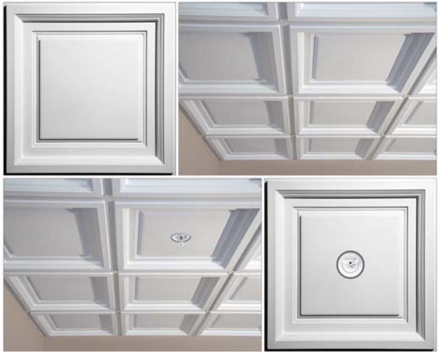
Sprinklers can be hidden above drop-out ceilings (top) or penetrate panels (below).
